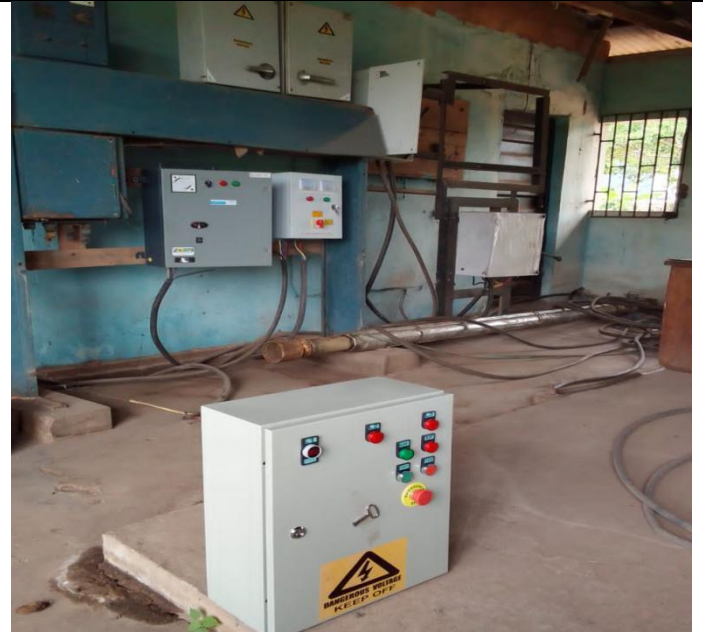
Installation of 25KW Starter
