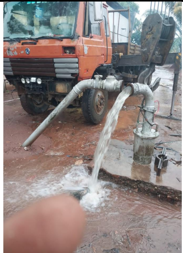
Testing of Water Flow in Umunede
